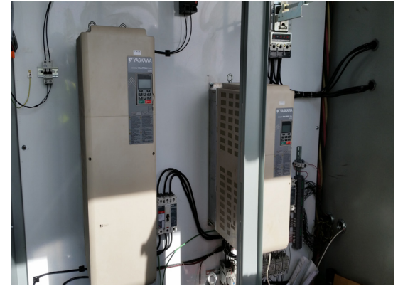
The U1000 Industrial Matrix drives significantly reduced the system complexity.
