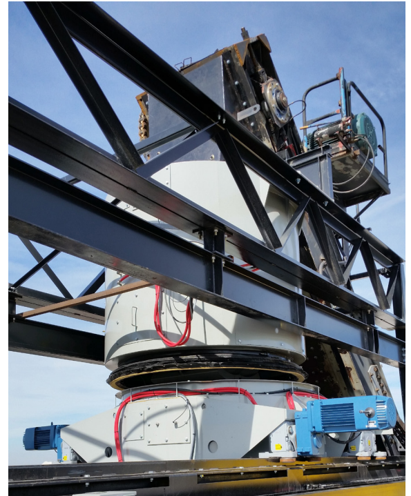
The system is designed to be more energy efficient and provide a more maintenance-free, mechanically integral distribution.
